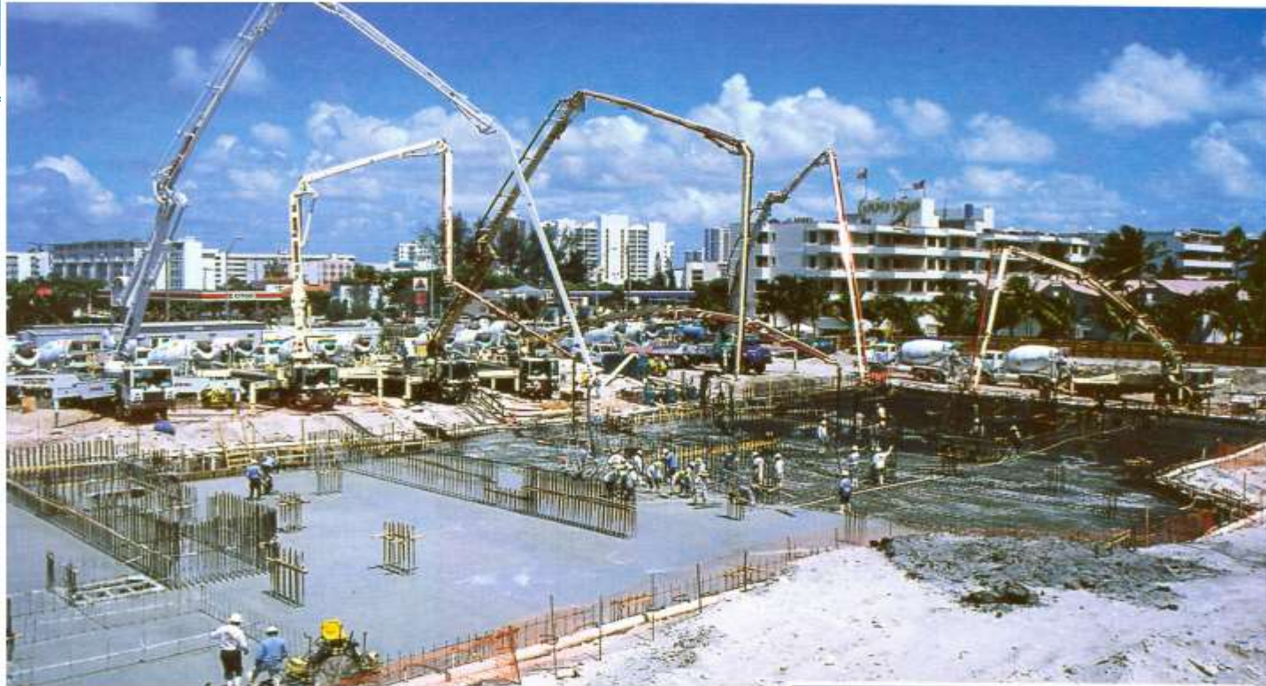
One of the largest mat foundations cast in Florida is this 9,900 yd 3 performed on Saturday, 11 May 2002, at Sunny Isles Beach, Miami. The mat supports the 51-story Acqualina Ocean Residences and Resort that belongs to the Trump Group. The pour took 14 hours (starting at 0300 hours to 1700 hours, non-stop).
