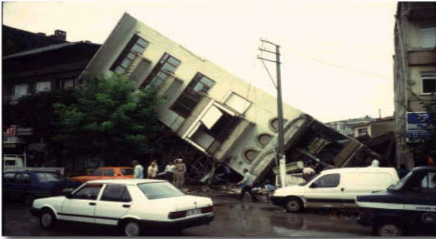
The Izmit, Kocaeli, Turkey earthquake of 17 August, 1999, liquefied the soil beneath this apartment building's shallow mat foundation by reducing the bearing capacity to zero.
